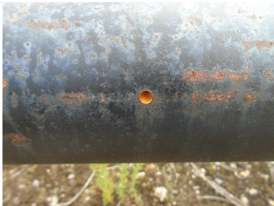
Image 3 4in pipe loop – Central Category 1 anomalous indication.
